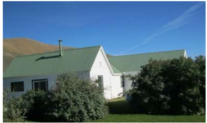
Photo 4. Detail of north and west elevations on the contributing farmhouse, view facing southeast.
